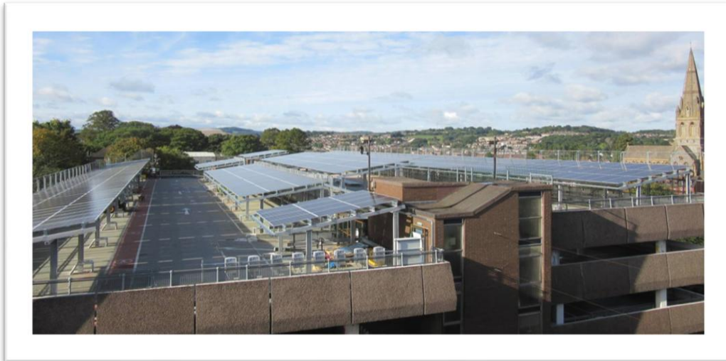
150kw array at Mary Arches Car Park
